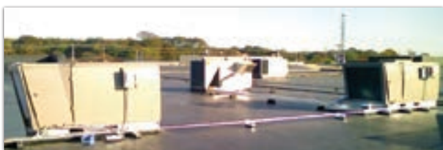
Ice Bear Installation on Roof of Big Box Retailer
