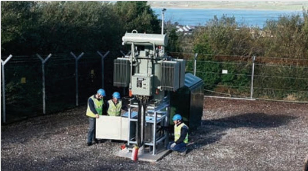
Arc Suppression System at Gurranbane Substation
