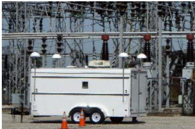
Figure 5-7 Antenna array installed on a portable trailer deployed in a 161-kV substation.
