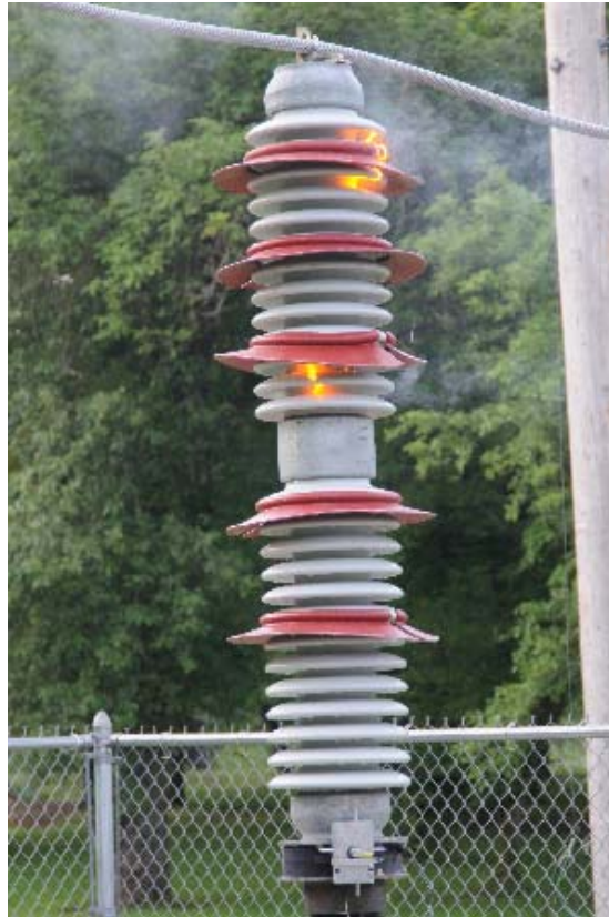
Figure 5-6 An RF leakage current sensor installed on a post insulator in a substation. It also shows dry band arcing (the discharge activity due to contamination and wetting that causes the leakage currents) captured during a contamination event. The sensor recorded the event
