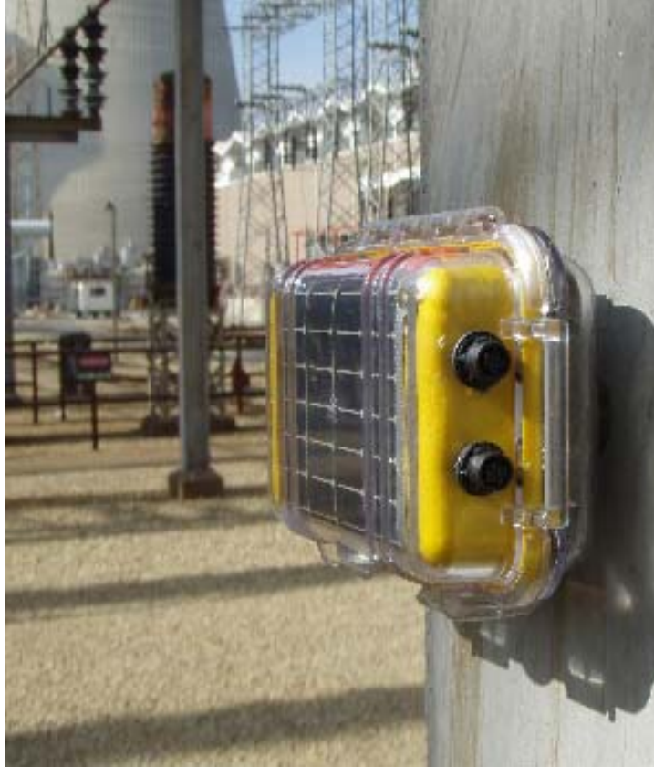
Figure 5-8 A solar-powered tank-top temperature sensor installed on a transformer.
