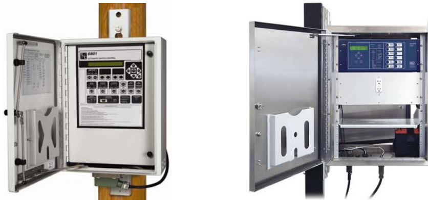
Figure 1. Examples of Automated Control Packages
